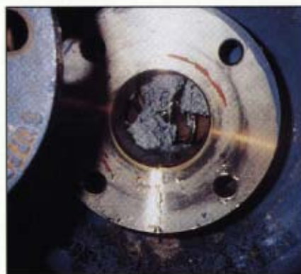
Top: Shortening of suction pipe was the only modification needed to fit the recessed-impeller pump where the conventional ANSI pump had been.
