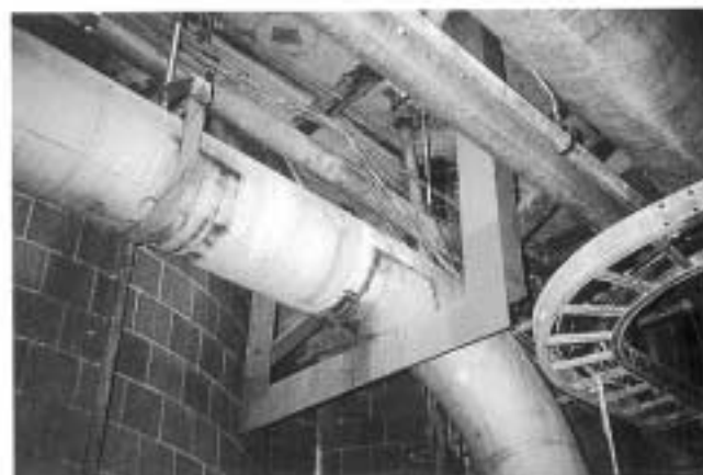
Figure 5. East Decker Piping System—Point C.
