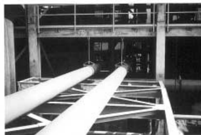
Figure 6. East and West Decker Piping Systems from Point E.
