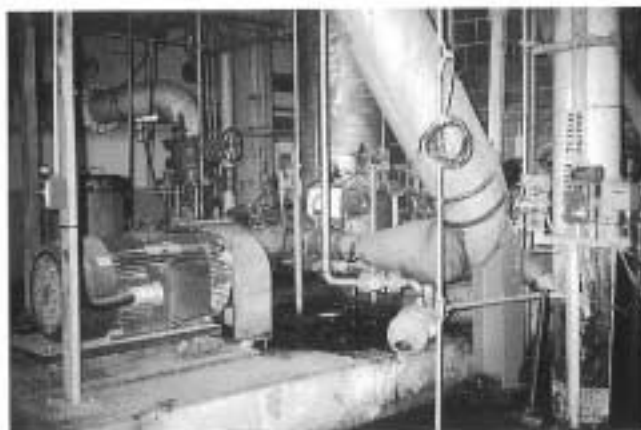
Figure 4. West Decker Pump, Standpipe, Control Valve, and Discharge Pipe.
