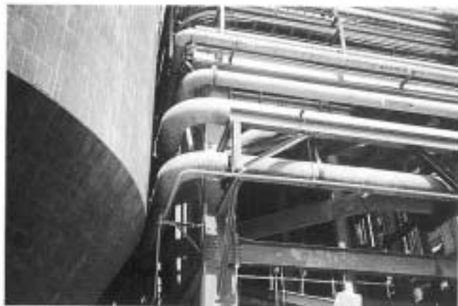
Figure 7. East and West Decker Piping Systems—Elbow Between Points F and G.
